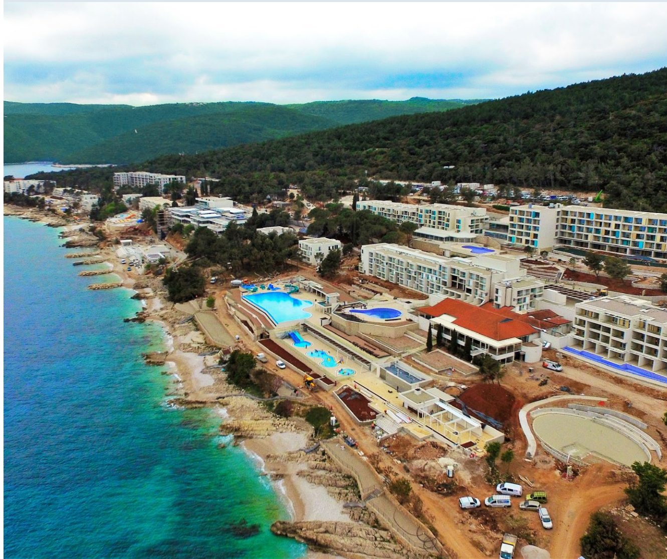
Interactive video footage of the construction site in Rabac on 24/4/2017 (Valamar Girandella Resort 4* and Family Life Bellevue Resort 4*), Rabac
